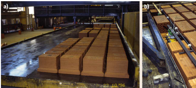
Fig. 57.8 (a) Automated horizontal brickwork layering robot station; (b) insertion of reinforcement and house infrastructure
