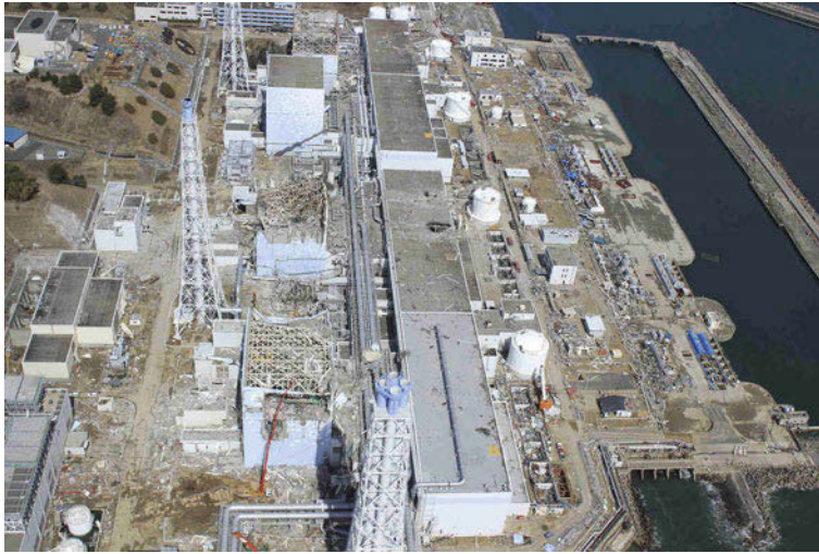
Fig. 58.21 Fukushima Daiichi Nuclear Plant after tsunami had inundated entire site to depth of over 13 m and subsequent hydrogen explosions. (courtesy of Japan Atomic Energy Agency)
